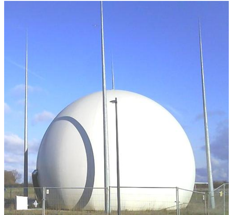
Biogas holder with lightning protection
